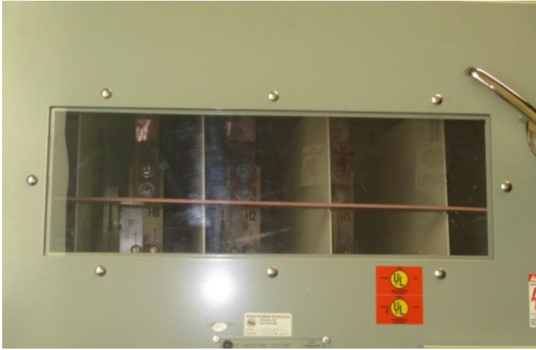
Figure 1 existing plexiglass window
