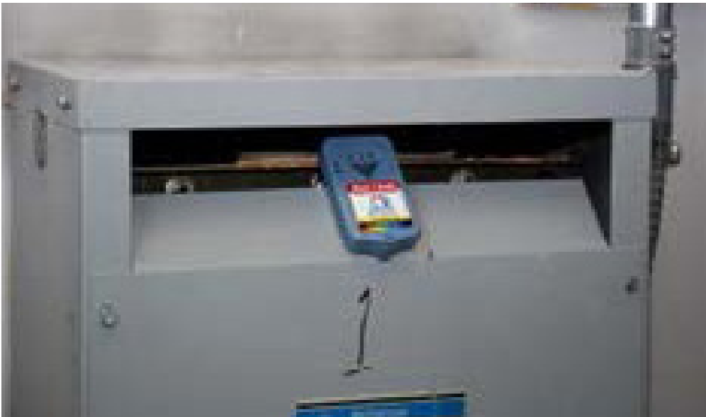
Figure 3 The Delta T Alert was magnetically installed on the vent of this transformer.
